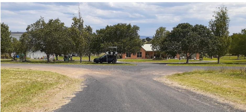
Photo 4: Anderson Street (north) approach to Flirtation Hill Lane – note loose gravel at the junction
