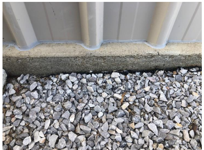
Figure 10 – Plastic membrane visible under slab edge
