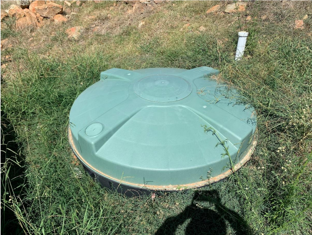
Plate 3 – Existing Plastic Standard Septic Tank
