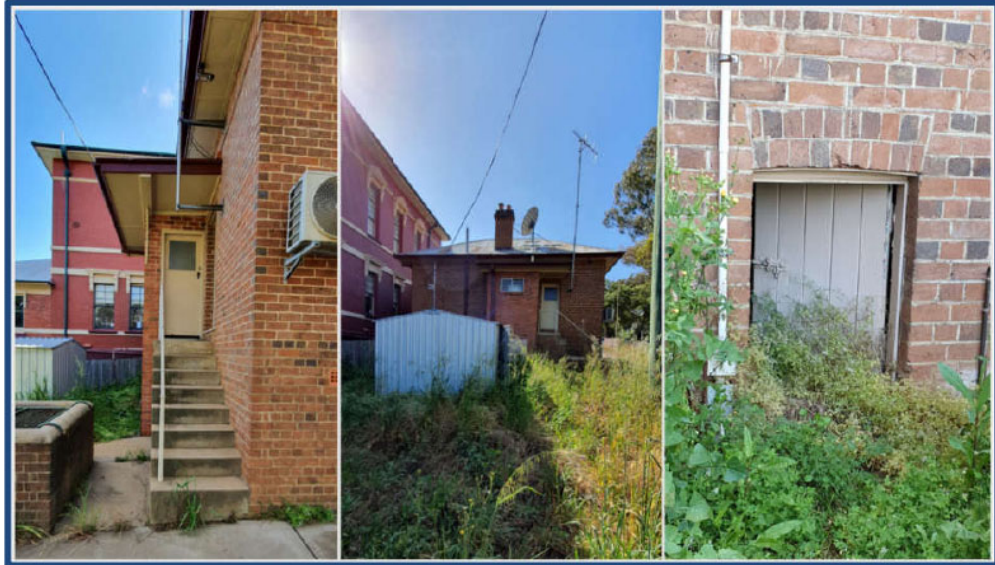
Figure 14 - Fire Station Rear (L-R) Rear entrance, rear view with garden shed, access to subfloor storage area.
