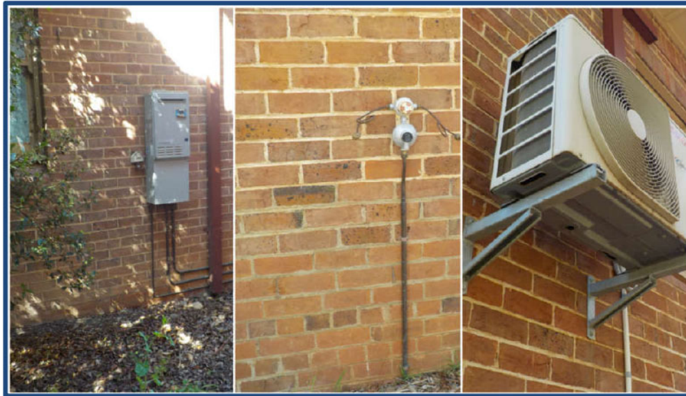
Figure 16 - Fire Station Installations
