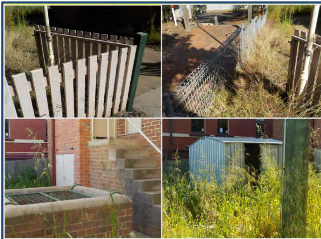
Figure 17 - Fire Station External Assets (Clockwise top LHS) boundary picket fencing and gate, fencing and path, garden shed and rear of Old Fire Station.
