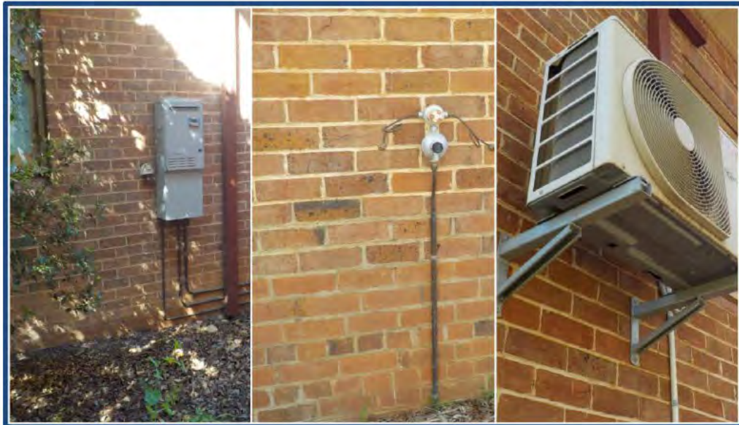
Figure 16 - Fire Station Installations
