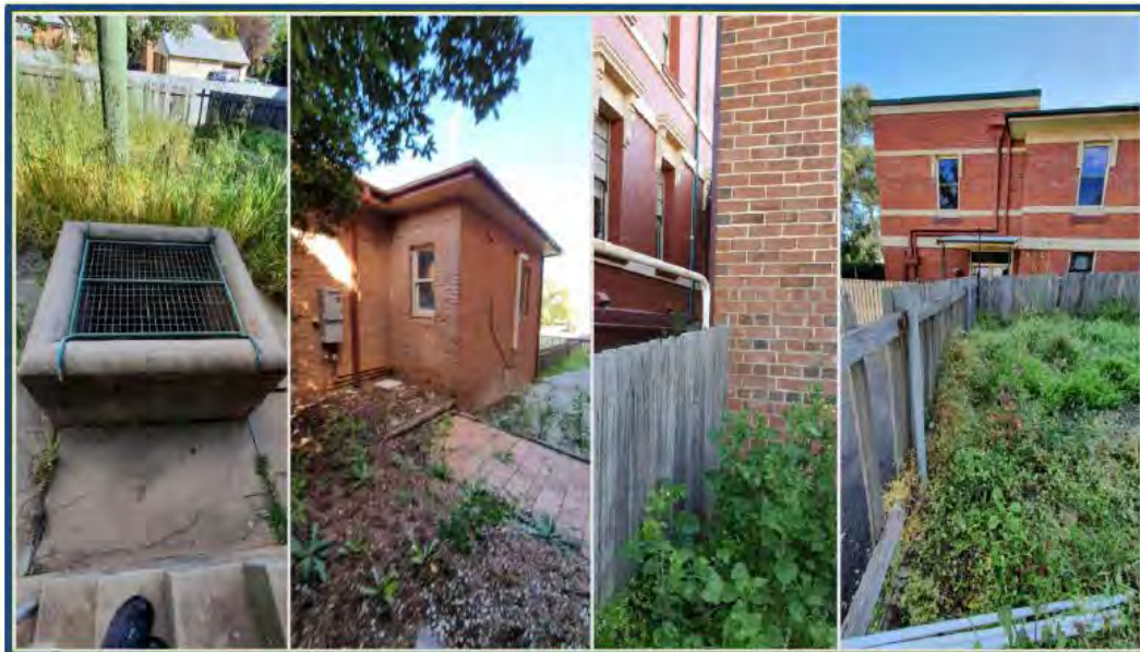
Figure 18 - Fire Station External Assets (L-R) Fire hose conditioning pit; NE aspect, main building; paling fence on boundary, NW corner building; back paling fence on boundary, viewing adjoining property to the north.
