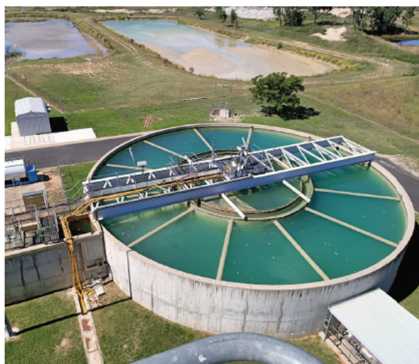
Mudgee Water Treatment Plant
