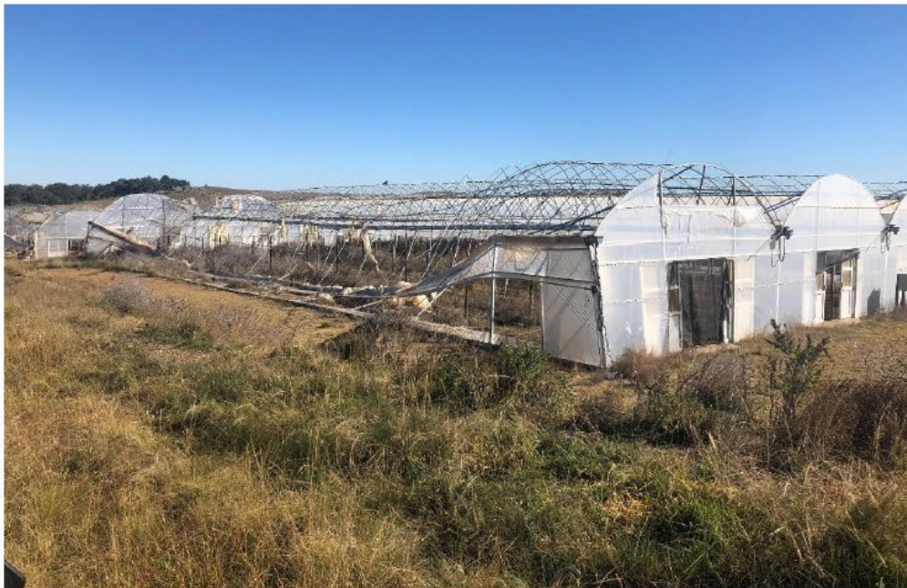
Figure 2.7: Picture from point F, showing disused and deteriorating greenhouses.
