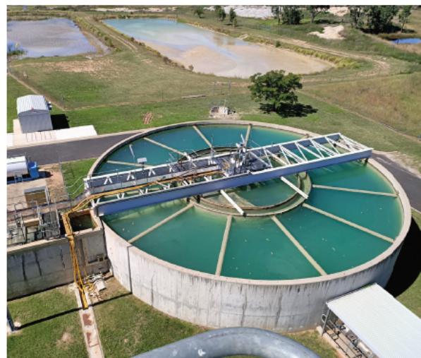
Mudgee Water Treatment Plant
