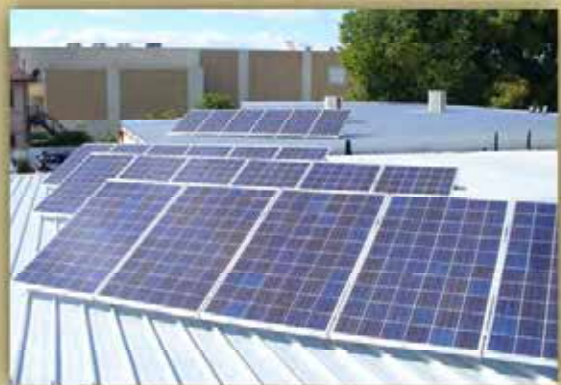
Solar array installed at Colemans Office Products
