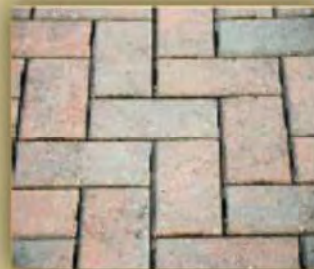
Permeable paving helps reduce runoff and pollutants from the site, helping to protect local creeks and streams
