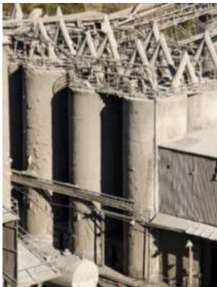
Figure 9: Concrete cement silos at the Kandos Cement works, part of the original works development in 1910's which were constructed using the slip-form method. Photo Karon Grant 2014
