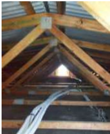
Figure 6: View showing the underside of the over-roof and the original concrete roof of the Kandos Museum (nave of the former Methodist Church). Photo credit Kandos Museum 2022.
