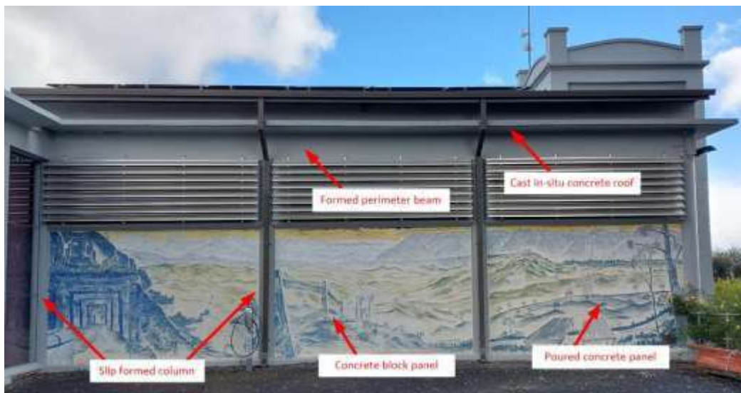
Figure 1: A view of the east wall of the Kandos Museum showing the primary structural elements of the nave. Photo credit Kandos Museum 2022.
