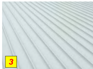
COLORBOND STEEL MATT ROOF
