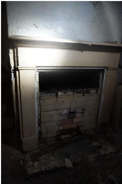
FIGURE 8 FRONT ROOM FIREPLACE AND SURROUND, FORMERLY BRICKED UP.
