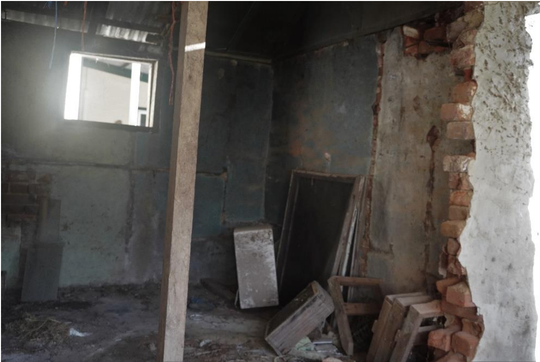
FIGURE 7 INTERNAL REAR ROOM SHOWING A PARTIAL COLLAPSE OF AN INTERNAL BRICK WALL: POSSIBLY A FIREPLACE.
