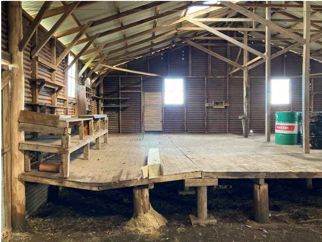
Plate 9 Raised workshop platform is in danger of collapse. Assorted post supports and random construction hint at a later period of construction from the main shed.
