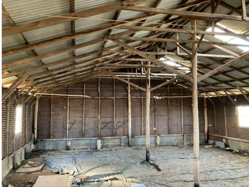
Plate 4 Interior of eastern section of machinery shed. Note earthen floor under plastic sheeting and use of farm sourced posts as uprights. Photo: Darrell Rigby 19.5.2022.
