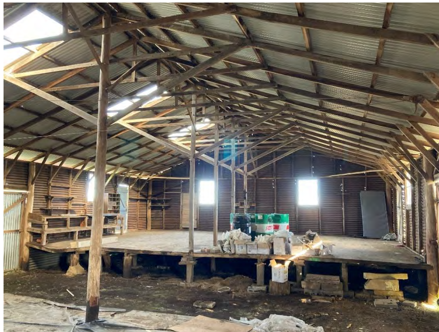
Plate 5 Western interior showing raised workshop area. Note collapsed platform section left of frame. Photo: Darrell Rigby 19.5.2022.
