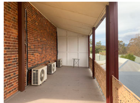
Figure 11: Southern verandah, looking east towards existing infill at first floor level. The proposed walk-in robe and ensuite are proposed to be contained within the existing verandah space along this elevation.
