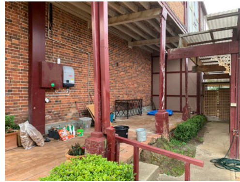
Figure 8: Southern verandah at ground level, looking east. The proposed kitchen, pantry, and lobby are to be located along this elevation.
