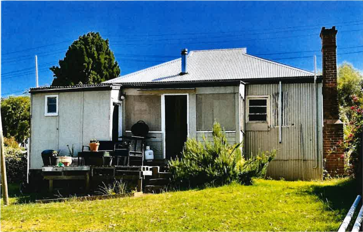
Figure 4: Figure 5 Rear view of residence showing hipped roof and chimney that will be retained. The small rear verandah, partially enclosed, and rear linings and wall will be removed. Image 13 December 22.
