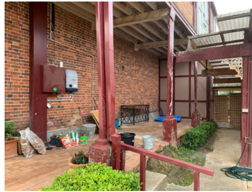
Figure 8: Southern verandah at ground level, looking east. The proposed kitchen, pantry, and lobby are to be located along this elevation.
