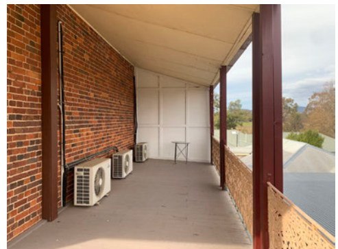
Figure 11: Southern verandah, looking east towards existing infill at first floor level. The proposed walk-in robe and ensuite are proposed to be contained within the existing verandah space along this elevation.
