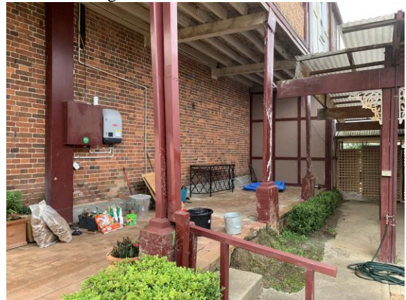
Figure 6: southern verandah, looking east. The proposed kitchen, pantry, and lobby are to be located along this elevation.
