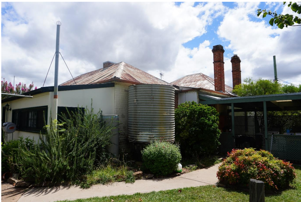
Figure 3 Rear view of residence showing hipped roof returns that have been infilled between, causing weatherproofing problems. Image 4 th March 22.
