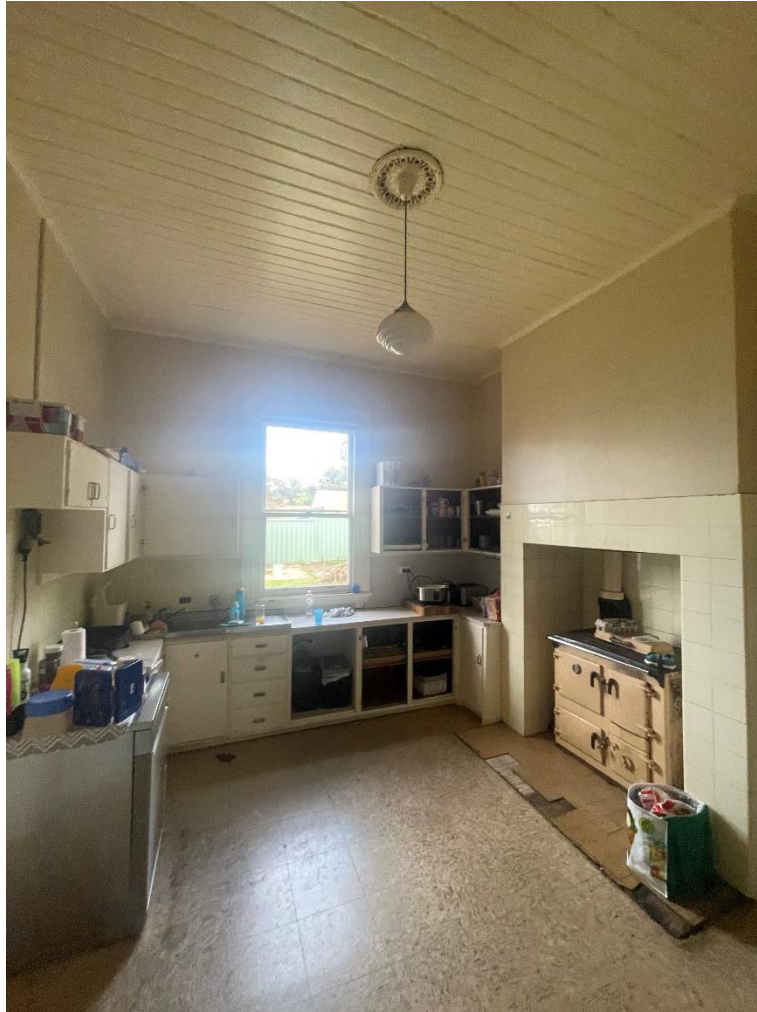
Figure 3: The Dilapidated Kitchen and Non-functioning Chimney
