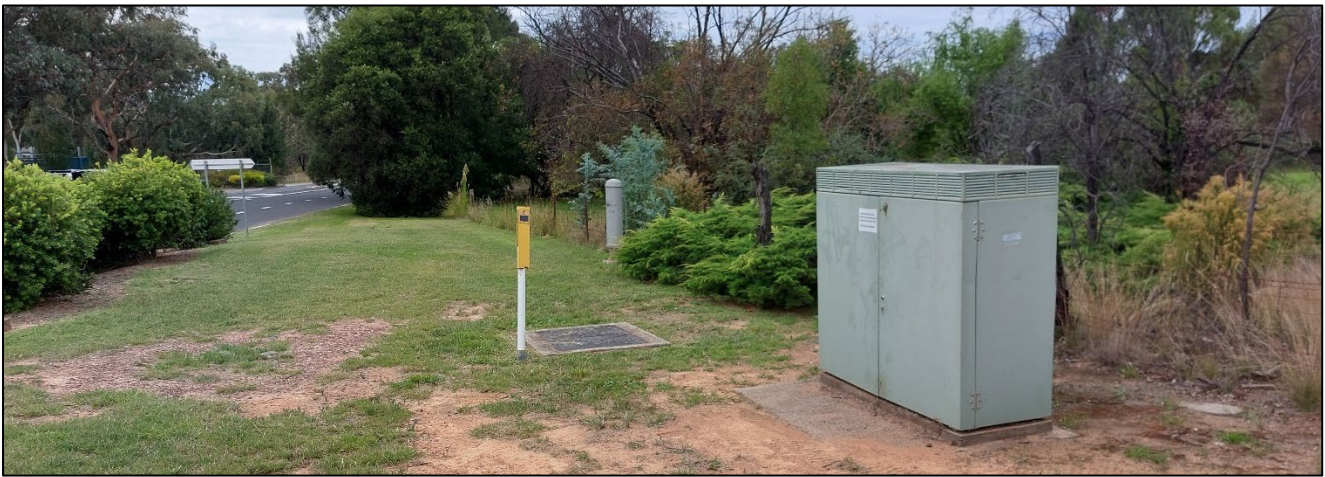
Figure 6. Existing electrical infrastructure on corner of Castlereagh Highway & Lions Drive
