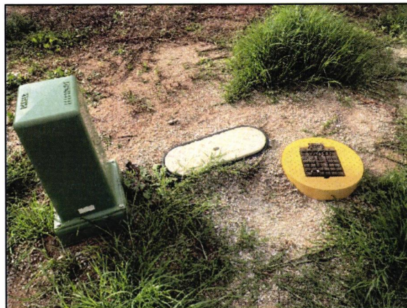
Photo 9: Services at rear of site.
