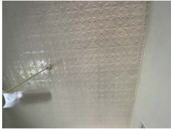
Figure 15: Detailed view of pressed tin ceilings.
