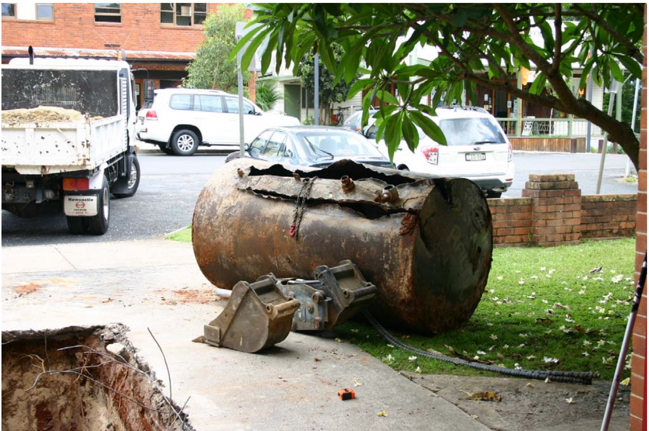
The tank after removal. The tank will be approximately 1.2m diameter and 2.2m long.
