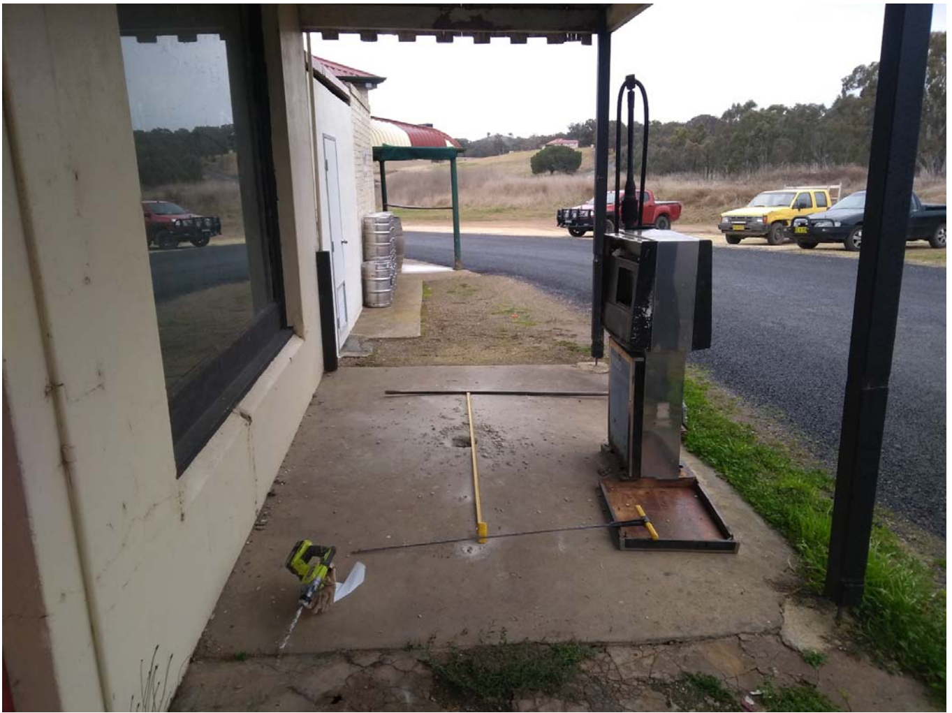
Photo showing position of the tank relative to the building. The tape shows the length of the tank and is located directly above the centre of the tank. The tank extends approximately 0.6m either side of the tape measure (as marked by the objects placed at either end of the tape). The tank pit will be approximately 0.5m from the façade of the building. The fuel dispenser will be situated very close to the tank pit, but will be removed prior to removal of the tank.
