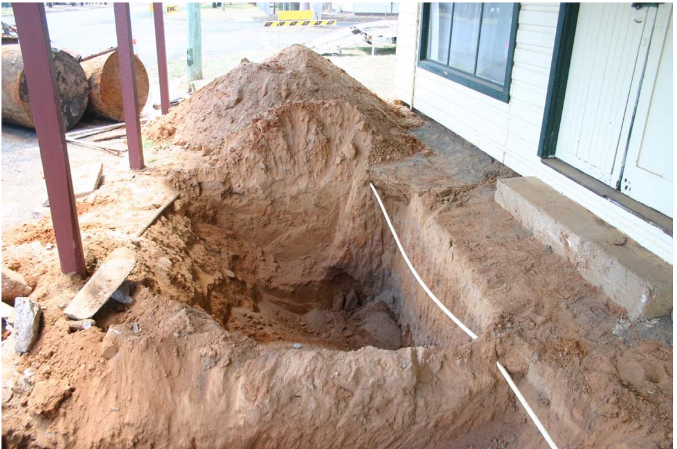
Excavations following removal of the tanks. A Telstra conduit was located over the ends of the tanks and was not damaged during the works.
