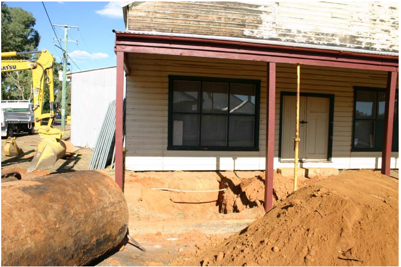
Photo showing limited clearance around the removed UPSS.
