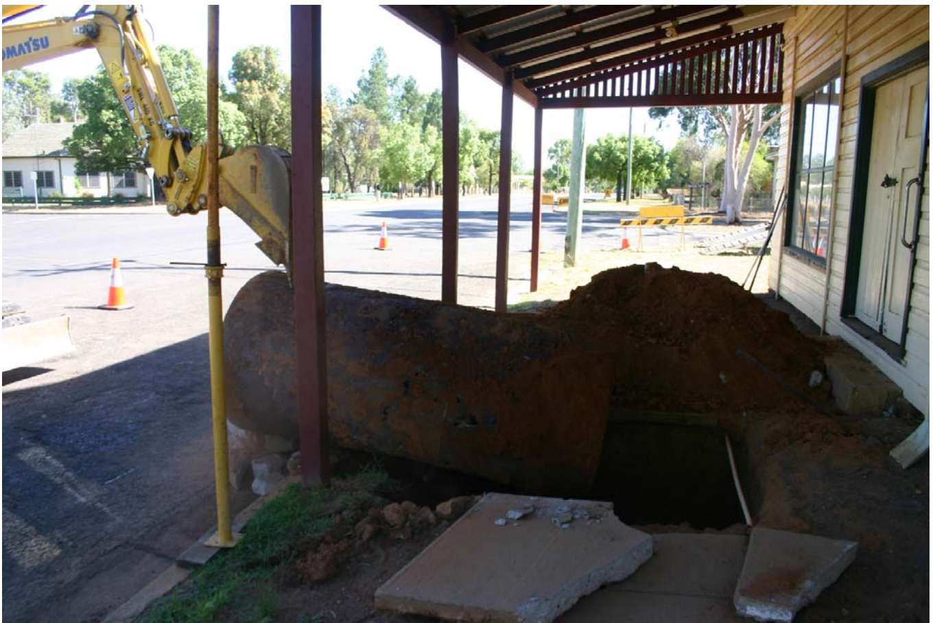
The awning was propped for added stability as the awning footing had potential to be undermined. The tanks were uncovered and carefully removed from beneath the awning
