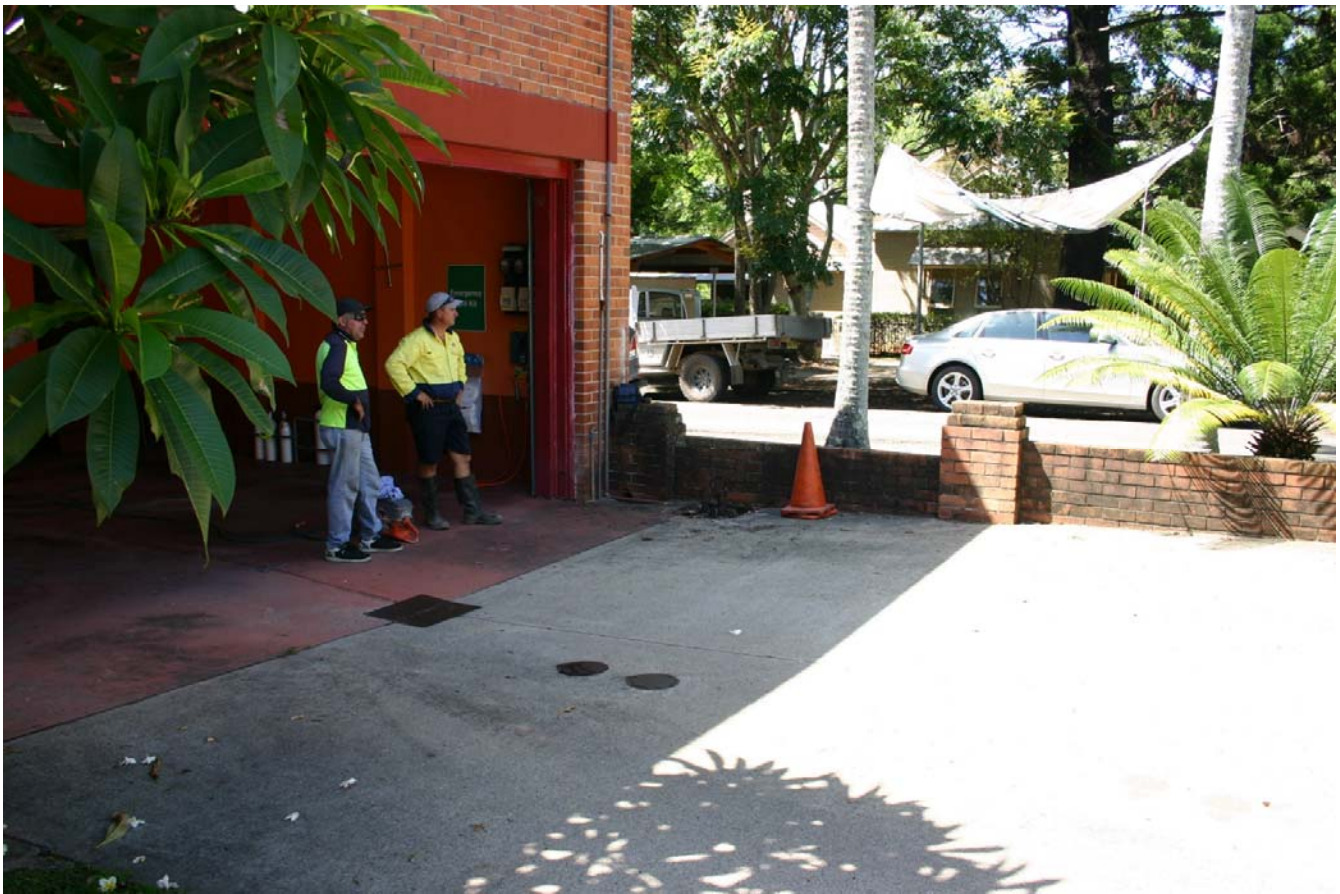
A 2200L tank at Bellingen Ambulance Station. The two steel lids in the driveway are the fill point and dip point for the tank. The tank at the proposed Lue Café has a single fill/dip point situated over the centre of the tank.
