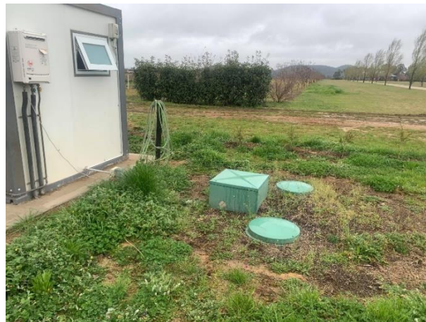
Image 1: Existing AWTS tank at proposed development site
